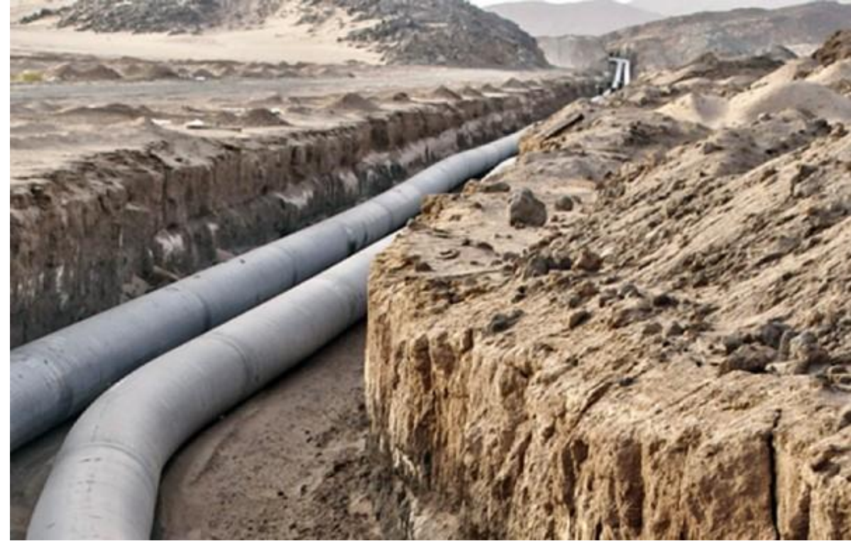
Water transfert In Salah -Tamanraset
